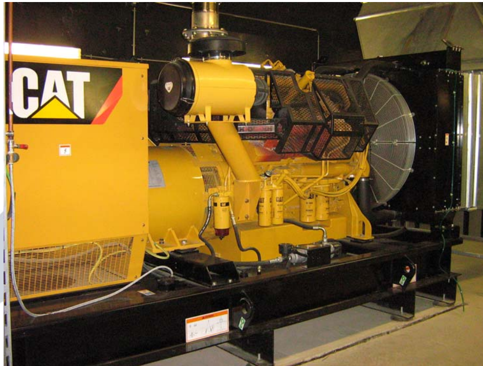
2 Diesel generators at ALBA
