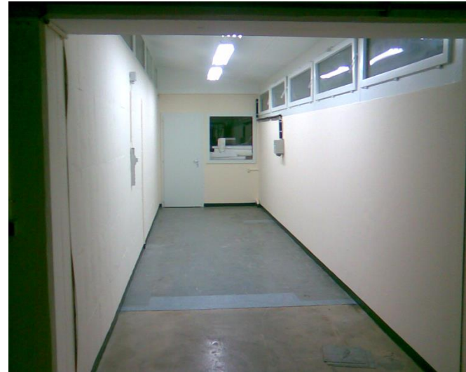
Old Workshop cleaned, painted and ready for the installation of the new mechanical and electrical/electronics workshop
