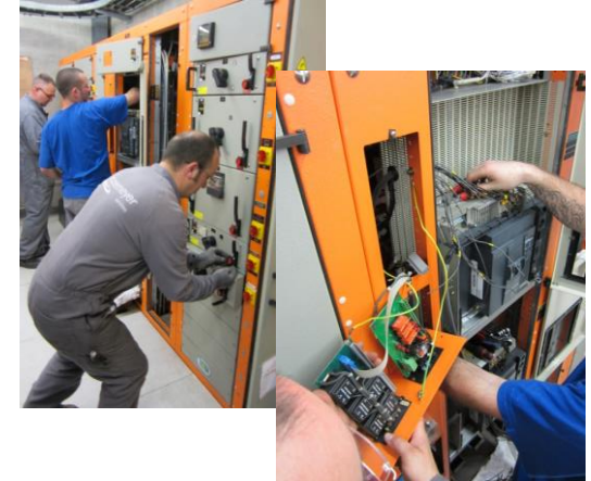
Electrical maintenance @ P8
