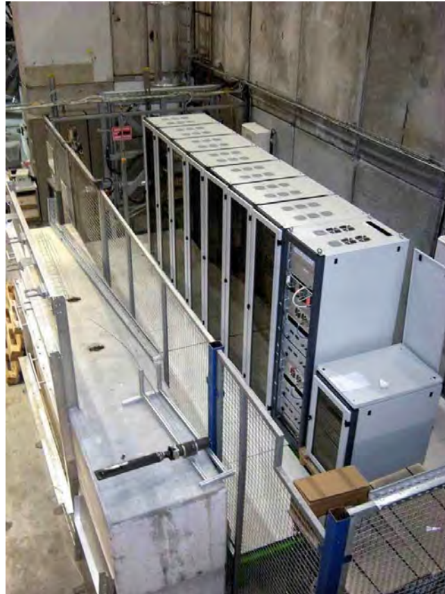
Fig. 37: Picture of the COMPASS polarised target control system installed in Bat. 888 (COMPASS experimental area).
