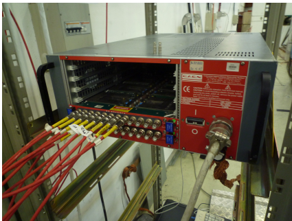
HV crate and modules
