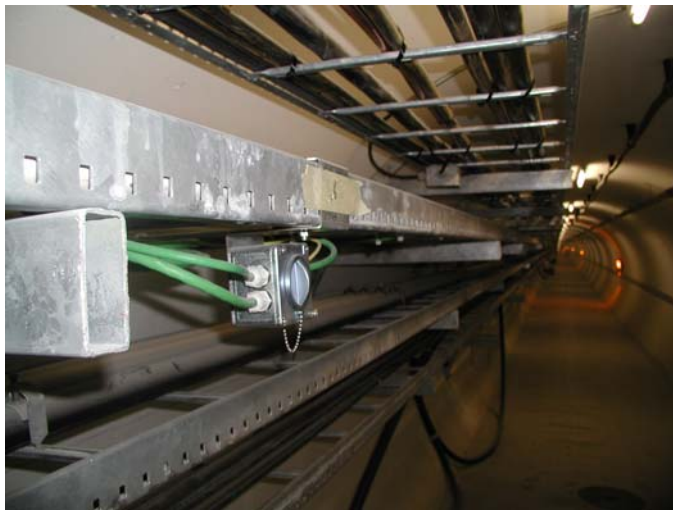
Junction box with signal cabling in ARC
