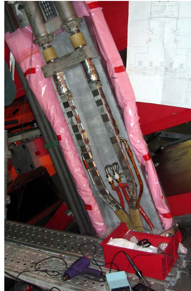
The current lead chimney assembly
