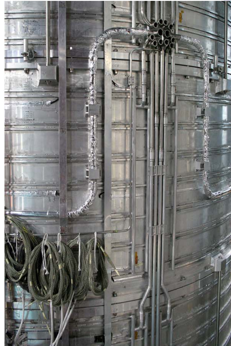
The cryogenic circuit closed to the chimney
