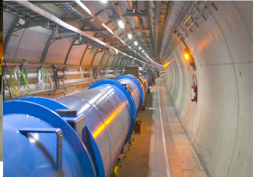
LHC tunnel - sector 81
