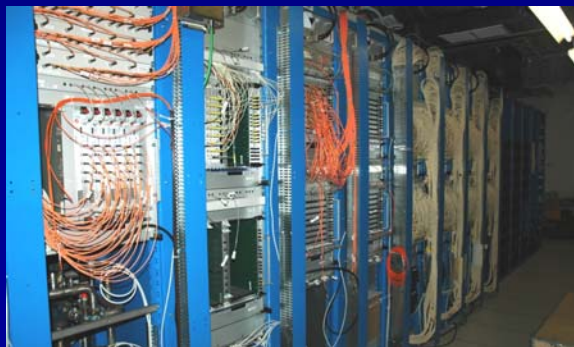
Optical fibers connected between FEBs and RODs
