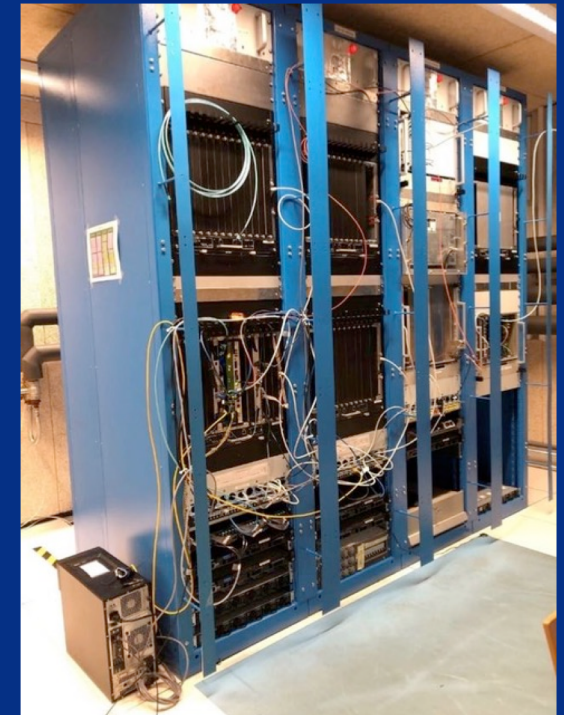
TDAQ surface test facility
