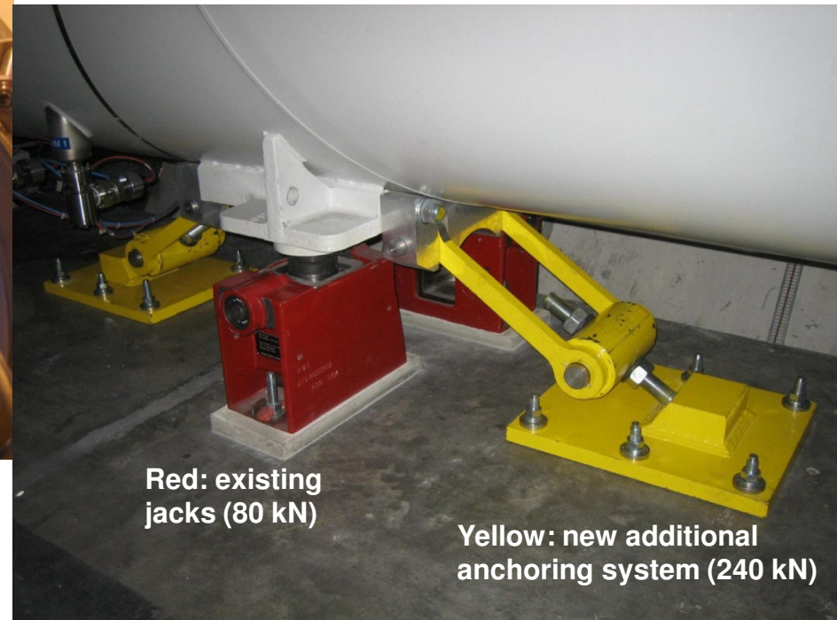
New additional anchoring system
