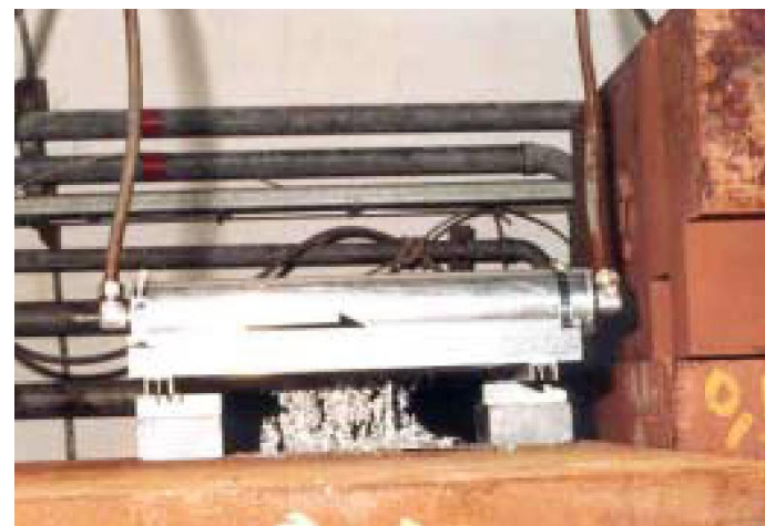
Lead block accidentally put into a p beam
