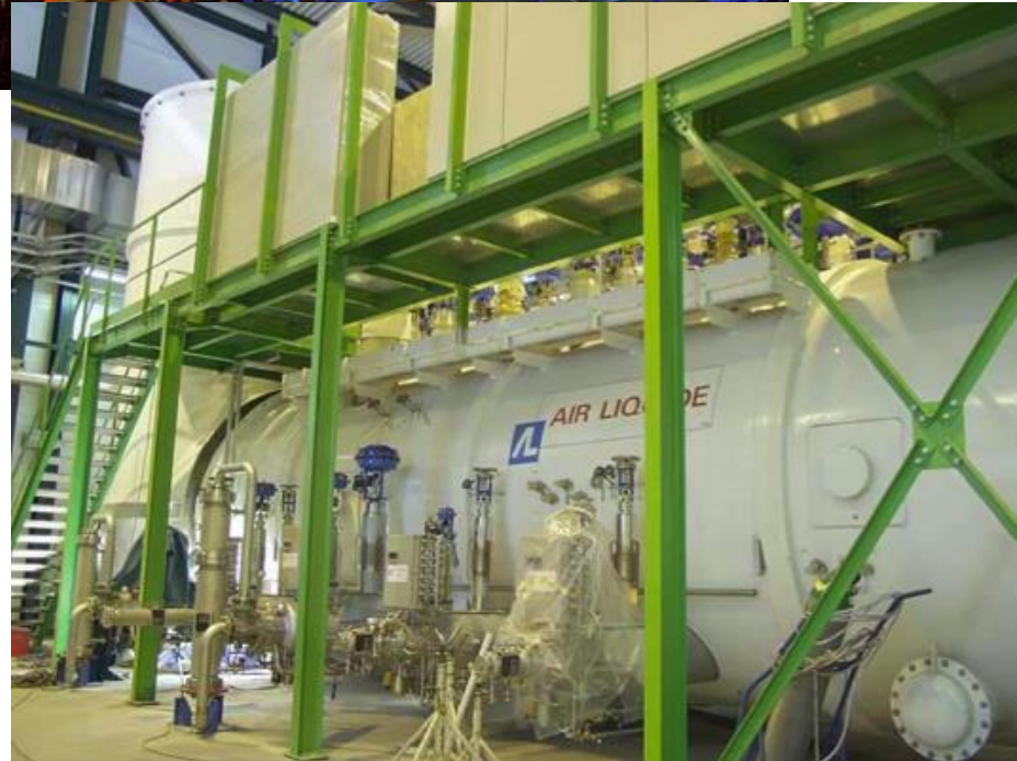
LHC refrigerators: \approx 140 \text{ kW @ } 4.2 \text{ K}
