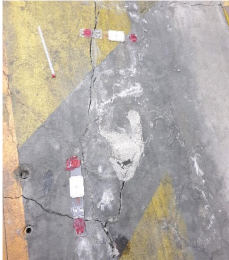
Monitoring equipment installed
