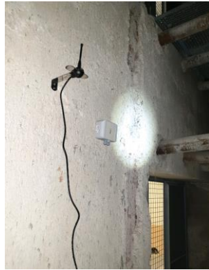
Extensometers (LHC P.4 headwall)
