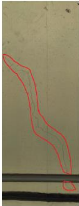
(a) Crack image
