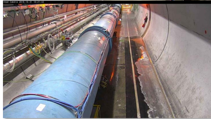
Example of water leak found by TIM2 during TS3 2018
