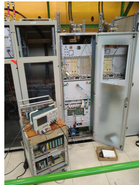
Test set-up in bldg. 180 (FAIR)
