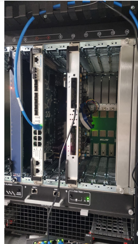
SerenityZ 1.1 with OpenIPMC-HW in the crate during STLink tests
