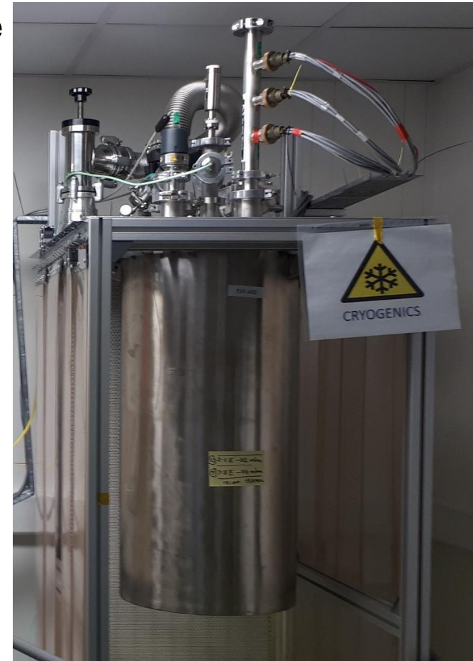
Pill-box cavity in a new facility with a closed-cycle refrigerator in STFC
