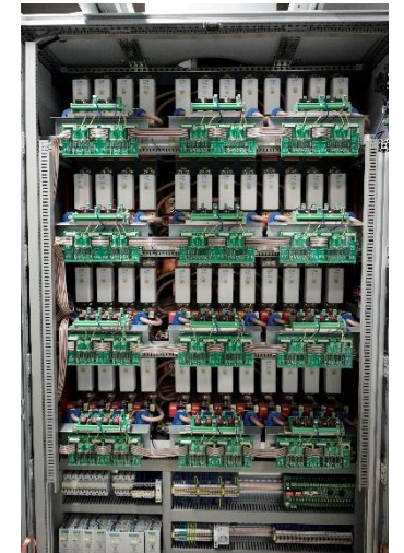
DC circuit breaker for s.c. magnet strings
