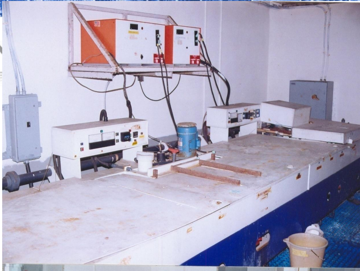
Plating line --- electrolytic gold
