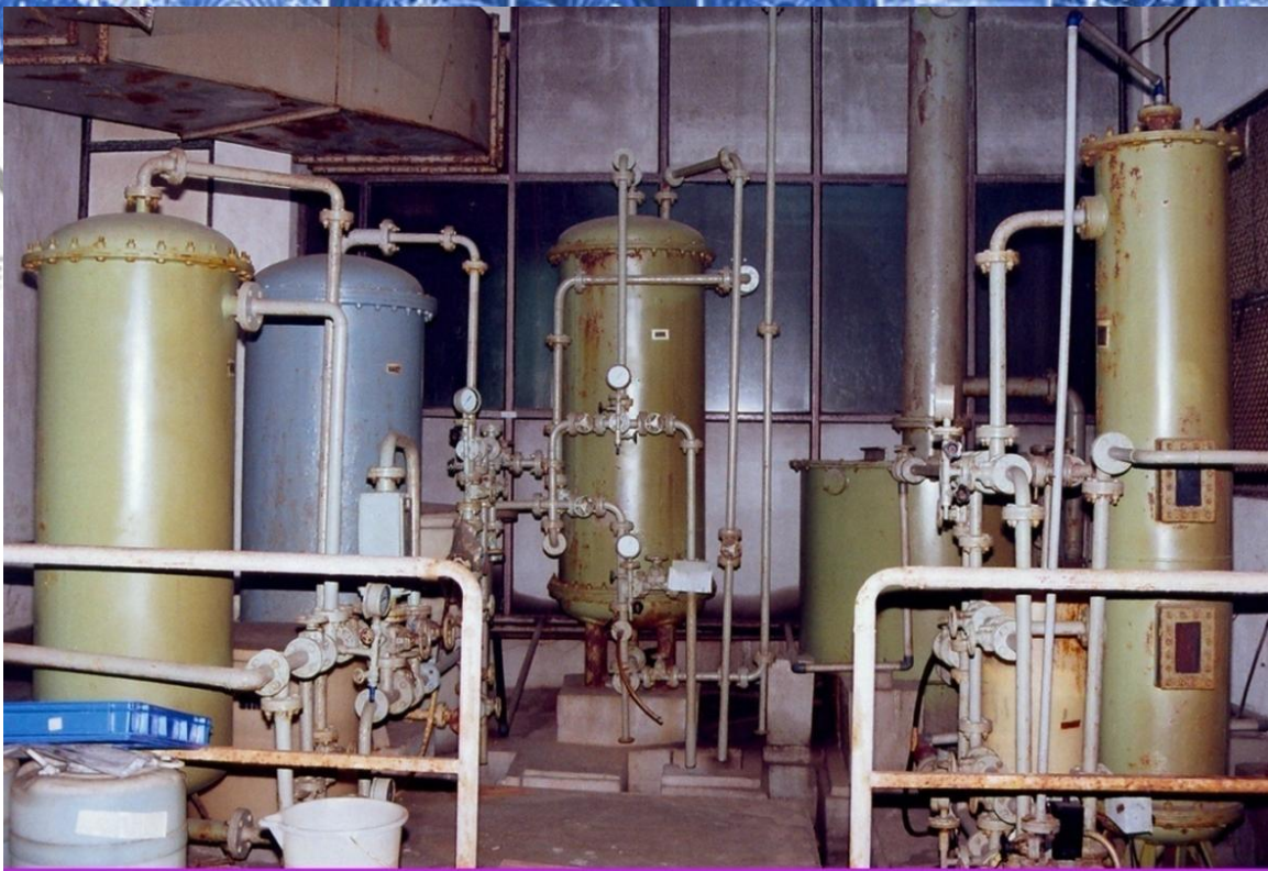
D.M. Water plant
