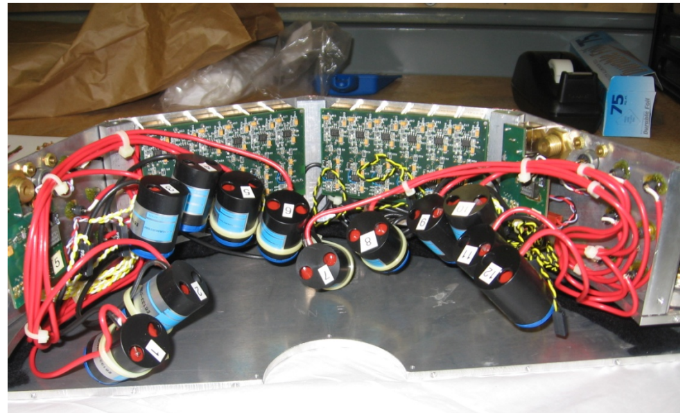
LM enclosure with the scintillator and PMTs removed during a maintenance period.
