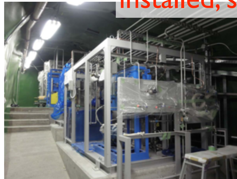
Xe extraction and storage line
