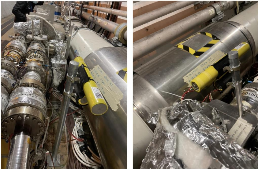
Installation in C4L8
