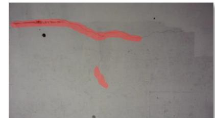
Example of crack found using vision based machine learning techniques
