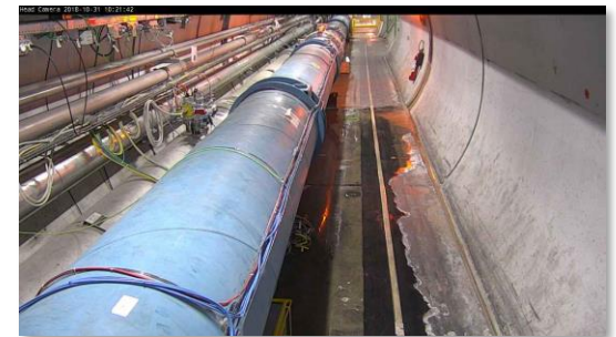
Example of water leak found by TIM2 during TS3 2018
