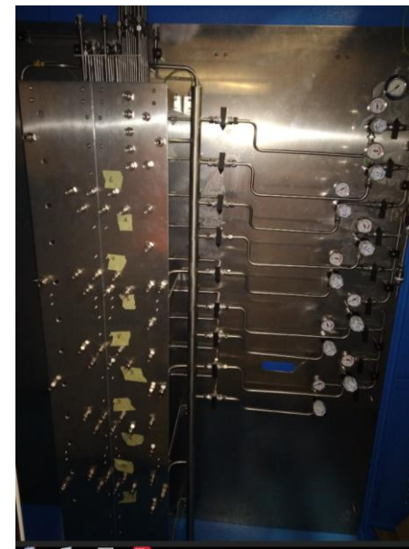
New gas distribution panel (and barrack) in 887/R-C47
