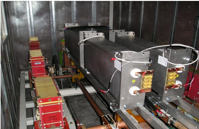
Figure 2 Snubber capacitors installed on a 13kA switch
