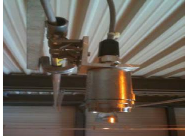
Figure 2: Oxygen deficiency gas sensor in the SD and SDx surface buildings.
