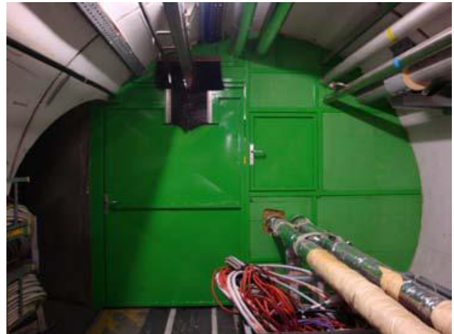
Figure 5: An example of "overpressure door" in the LHC machine
