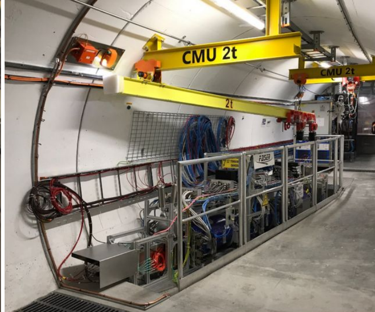
April 2021, BSM search detector fully installed
