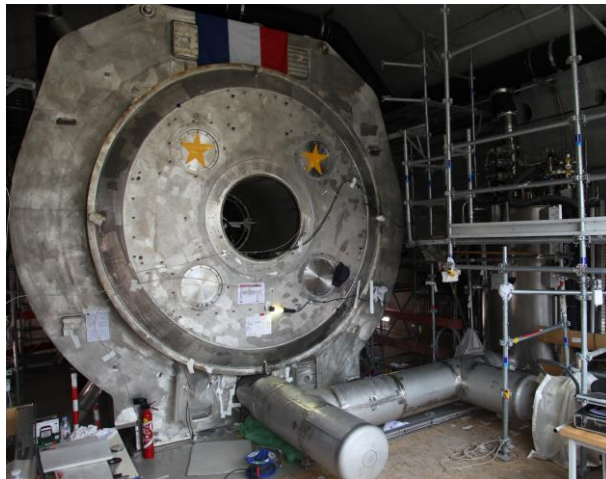
Iseult - On-going commissioning CEA Neurospin - France
