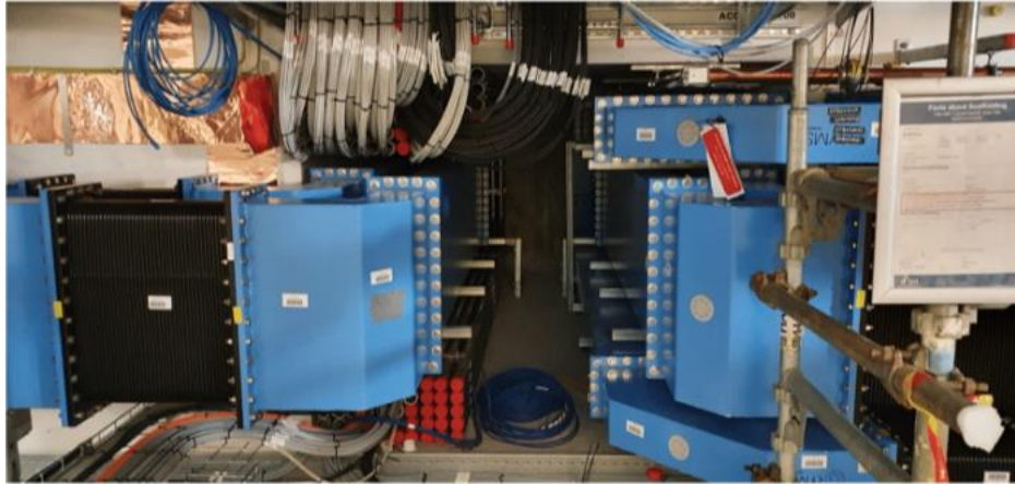
NCL RFDS, Tunnel
