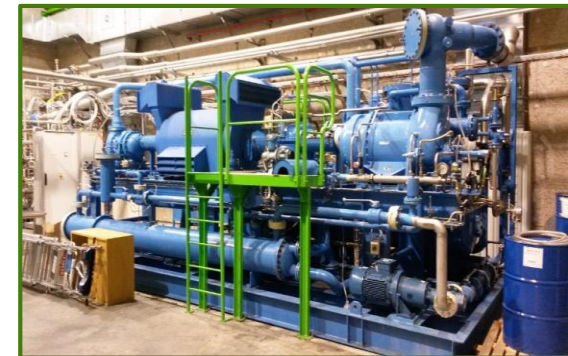
HIE ISOLDE Compressor station
