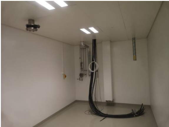
Carburization area (separated from power supplies room)
