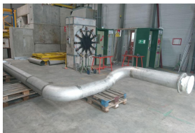
The new ^3\text{He} pumping pipe.
