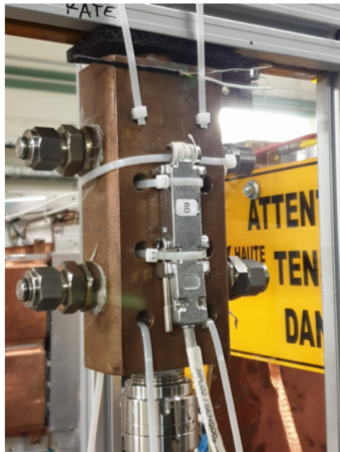
EN-CV : tightness of cooled cables manifolds
