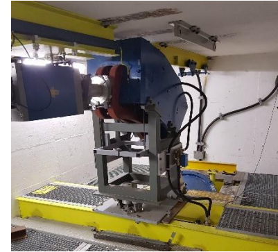
Beam delivery system
