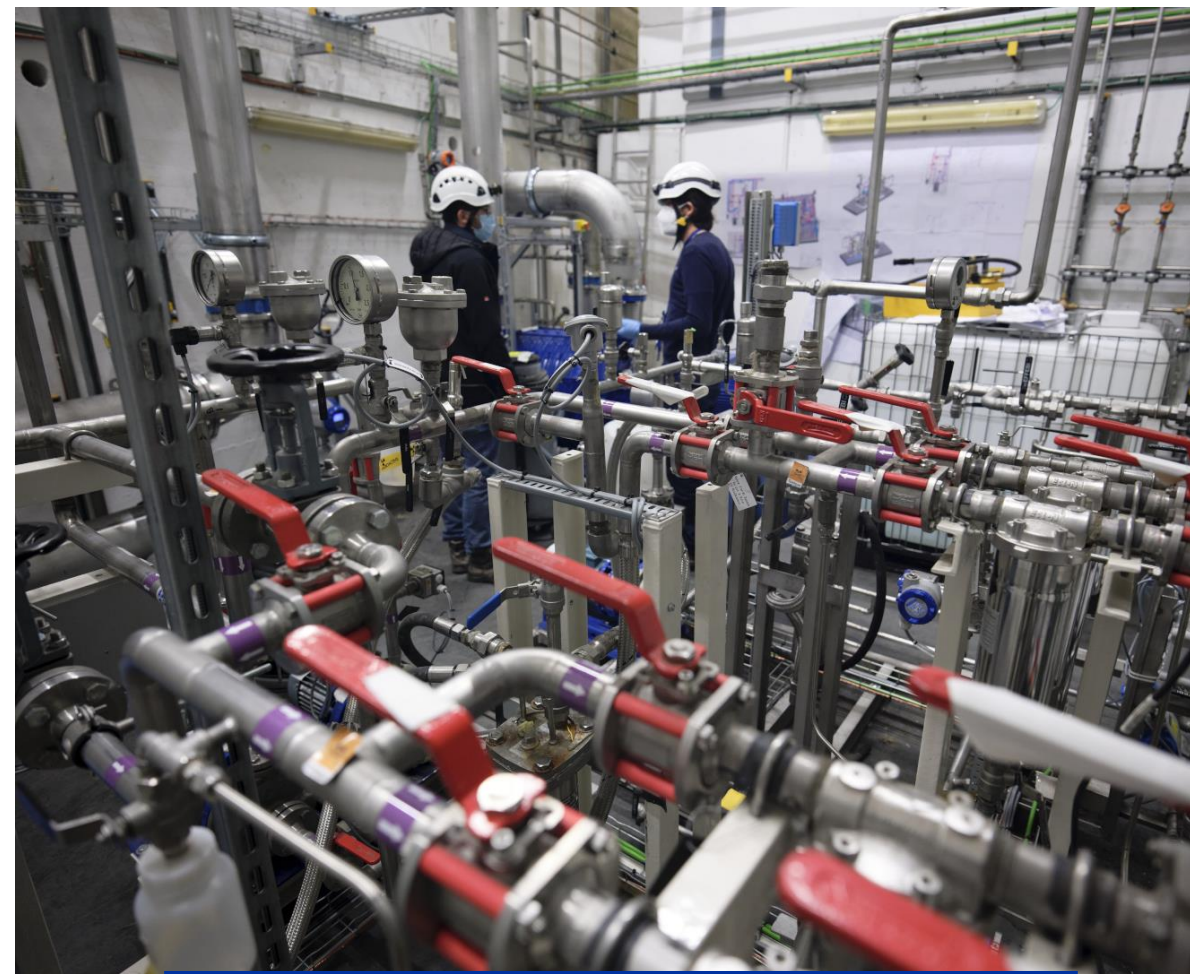
Cooling and moderator station
