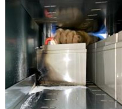
UPS battery fire outbreaks
