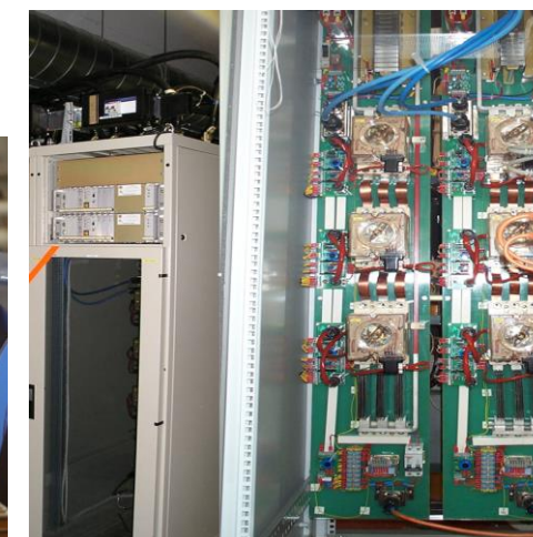
600A EE system maintenance
