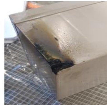
UPS battery fire outbreaks
