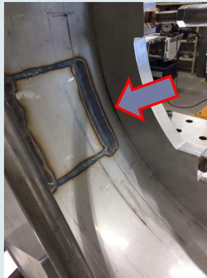
Closeup showing deformation caused by the weld
