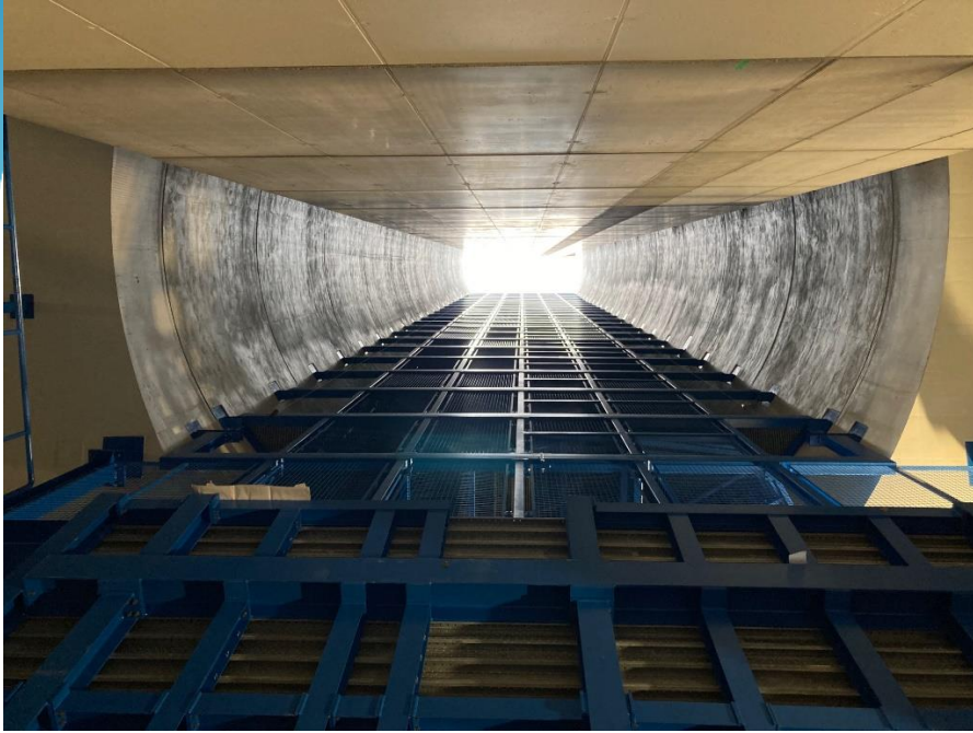
PM17 shaft equipped with concrete modules and metallic structures
