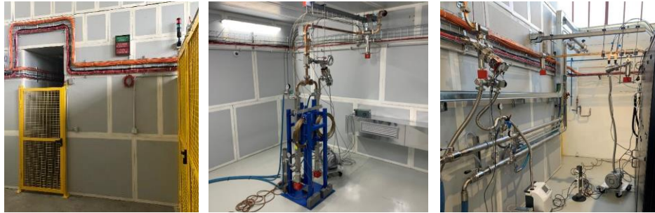
Concrete Bunker and Modulator Cage with the RF Source
