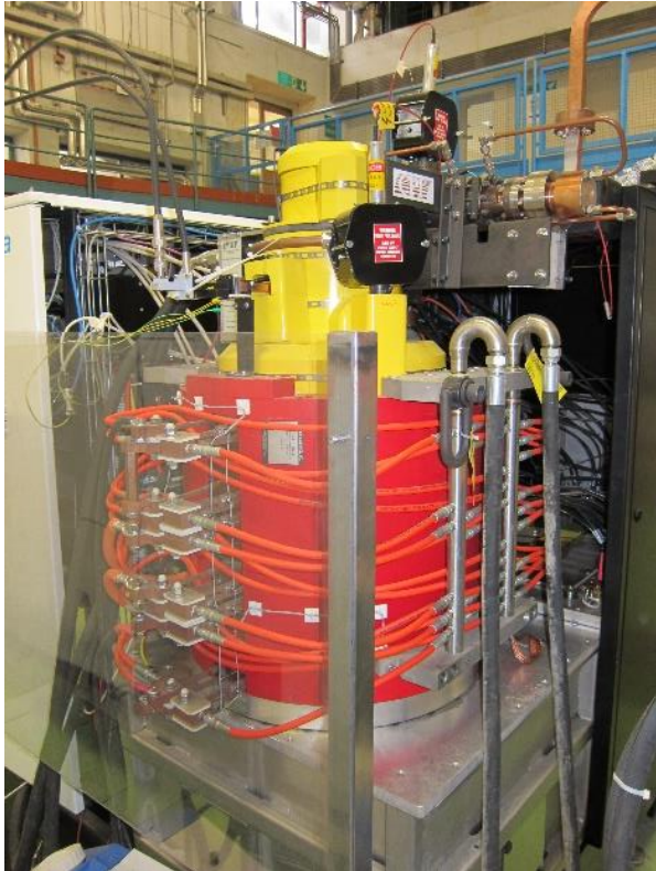
Existing commercial CPI 50 MW klystron in Xbox-2
