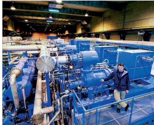
LHC warm compressor station
