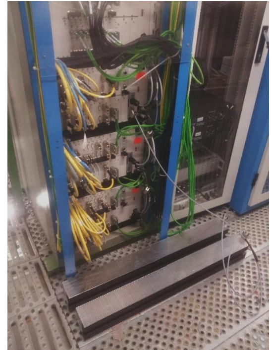
Remote online tests and PLC tests.
