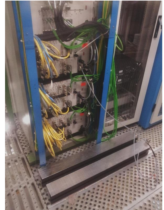
Remote online tests and PLC tests.
