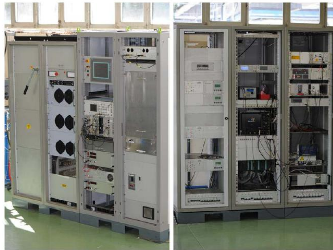
Figure 35: Left: High voltage and 2MHz RF generator. Right: Vacuum and controls racks
