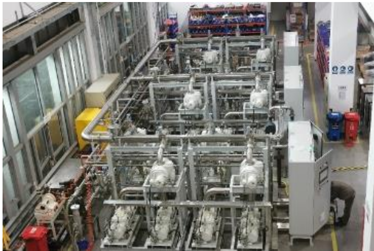
Cryogenic system hall in 2020
