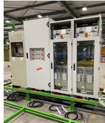
Cluster-F installation 2 x 2 kA EE systems
