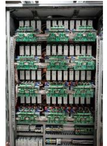
DC circuit breaker for s.c. magnet strings
