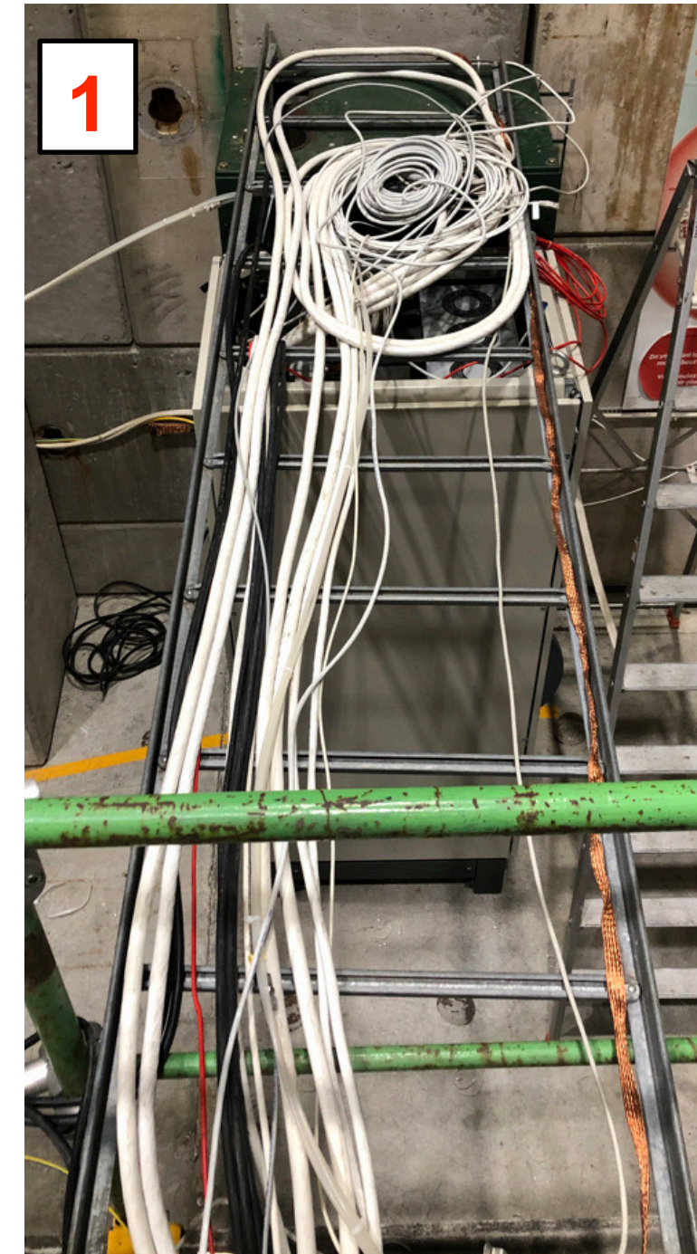
Cables for PLC
