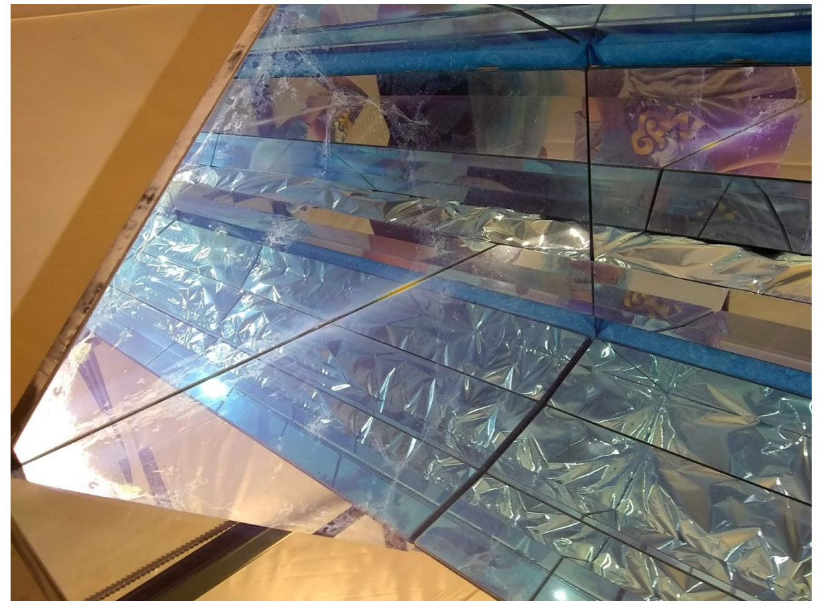
Residue on mirrors after commissioning
