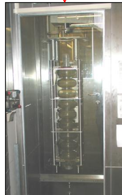
DESY's HP rinsing system
